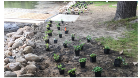
Pots are already for planting to create a buffer zone and the new post dock is installed replacing the old crib dock.
